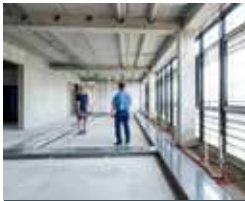
OKA underfloor installation trunking
