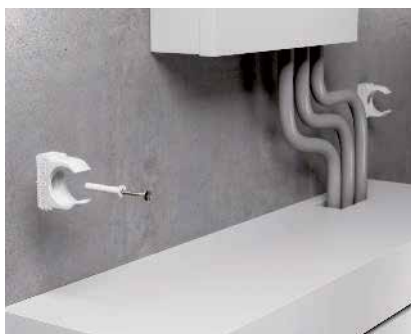
RK clip mounting The clips (OBO Quick clip Pg16) are mounted using knock-in anchors on the left and right of the switching cabinets. The knock-in anchors are contained in the scope of delivery.
