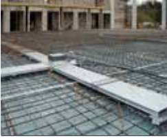
In-concrete duct system
