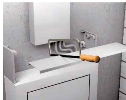
Cutting RK covers The covers are cut to the appropriate length using a standard coping saw.
